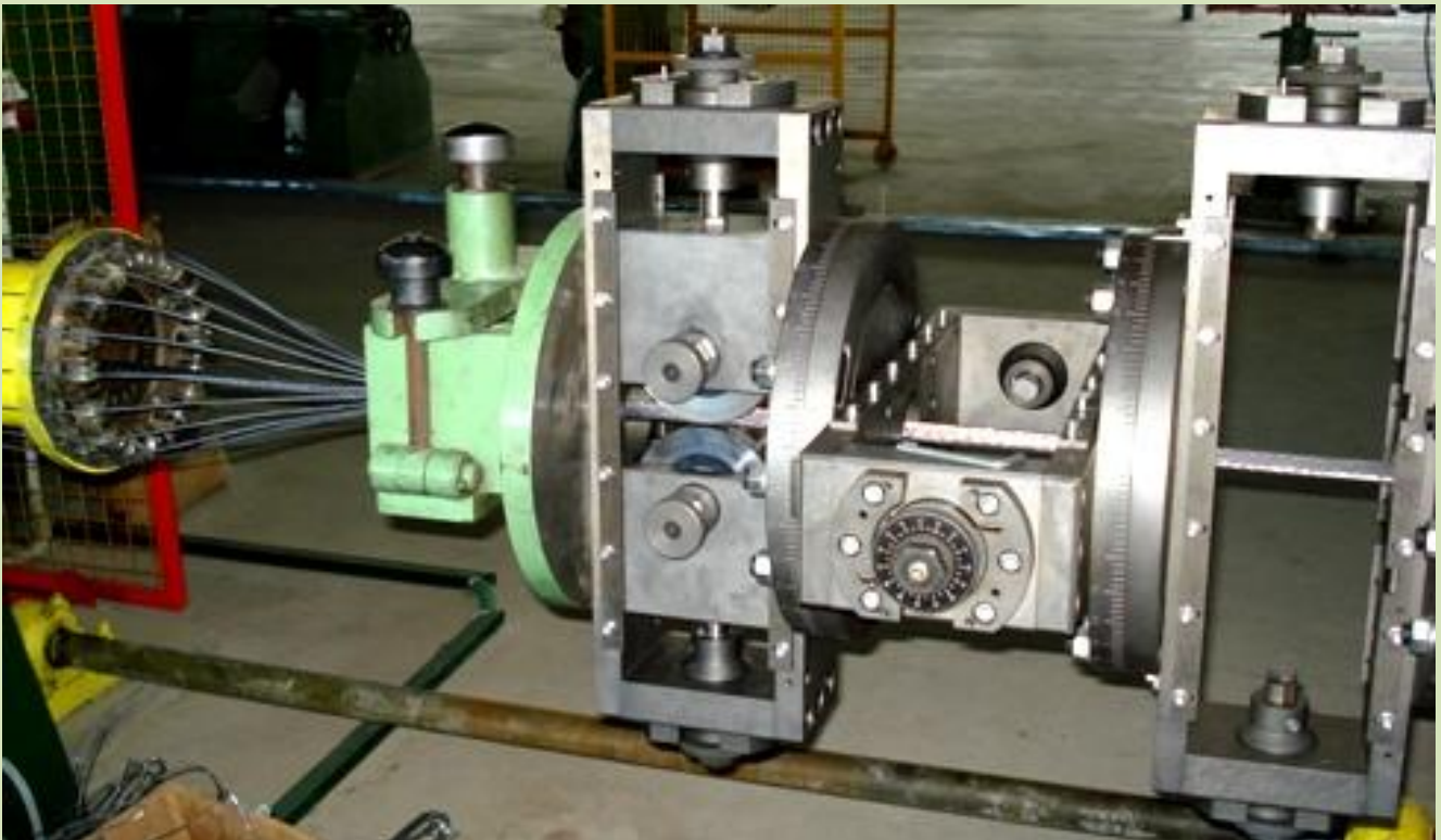
The all part of line are old. Upgrading is only Pourtier's design the holders of rollers (CASSETTES)
